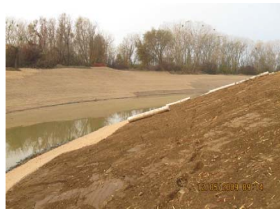
Feather Setback area drainage swale
