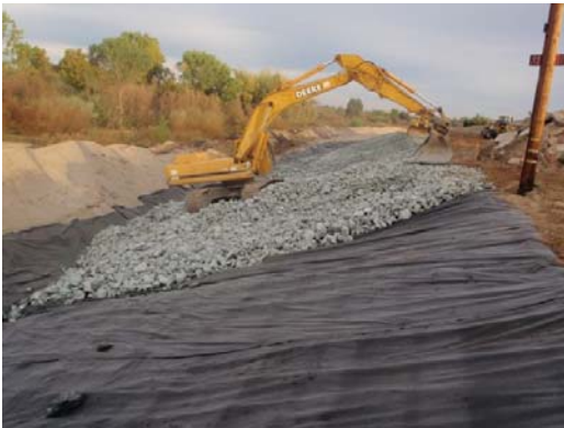
Erosion Site 2 – Feather Segment 3
