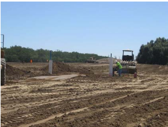
Inclinometers @ South Tie-In Cultural Site
