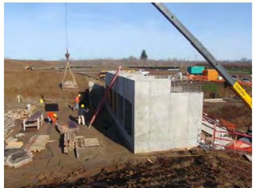
February New Pump Station # 3
