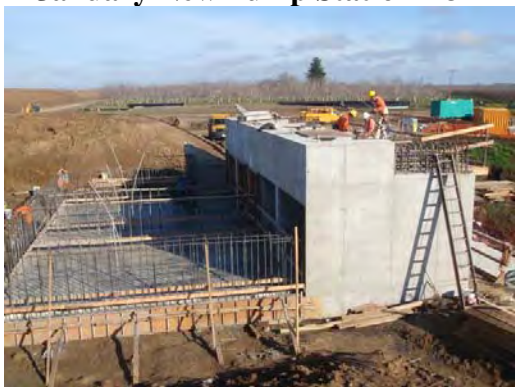
March New Pump Station # 3
